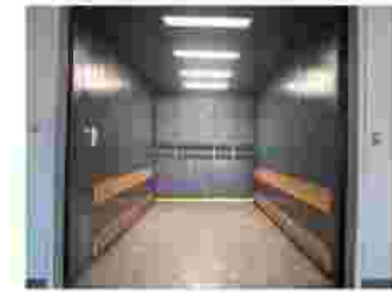
Freight lift to transport heavy goods to different floors.
